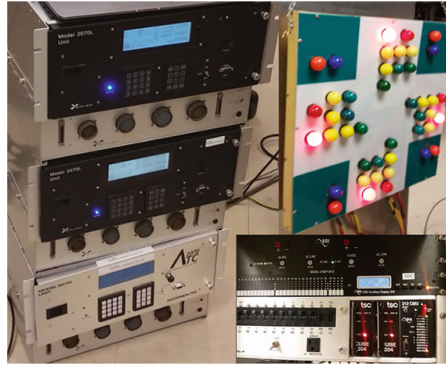
Fig. 3. Traffic Signal System in the municipality test lab. The left side shows a group of Model 2070 ATCs. The right top of the figure shows the traffic signal bulbs while the right bottom of the figure shows the CMU-212.
